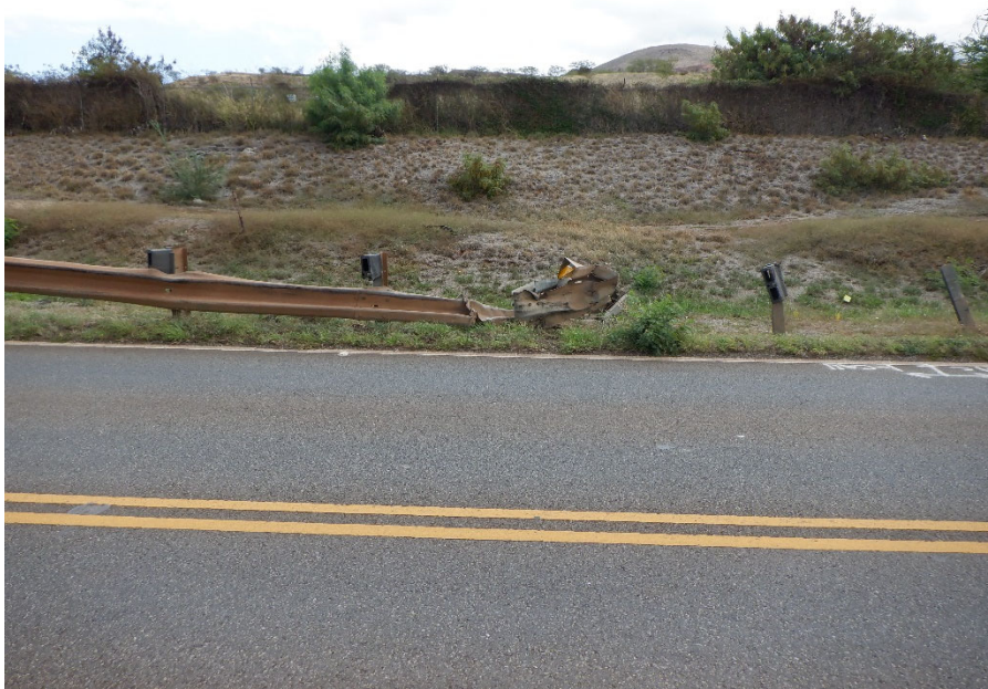
PHOTO 9 COLLISION DAMAGE TO UPSTREAM NORTH APPROACH GUARDRAIL AND END TREATMENT
