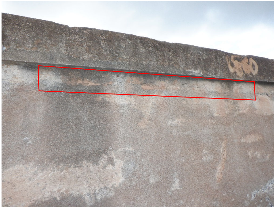
PHOTO 14 DELAMINATION (8FT 1080 CS2) ON EXTERIOR FACE OF UPSTREAM RAILING
