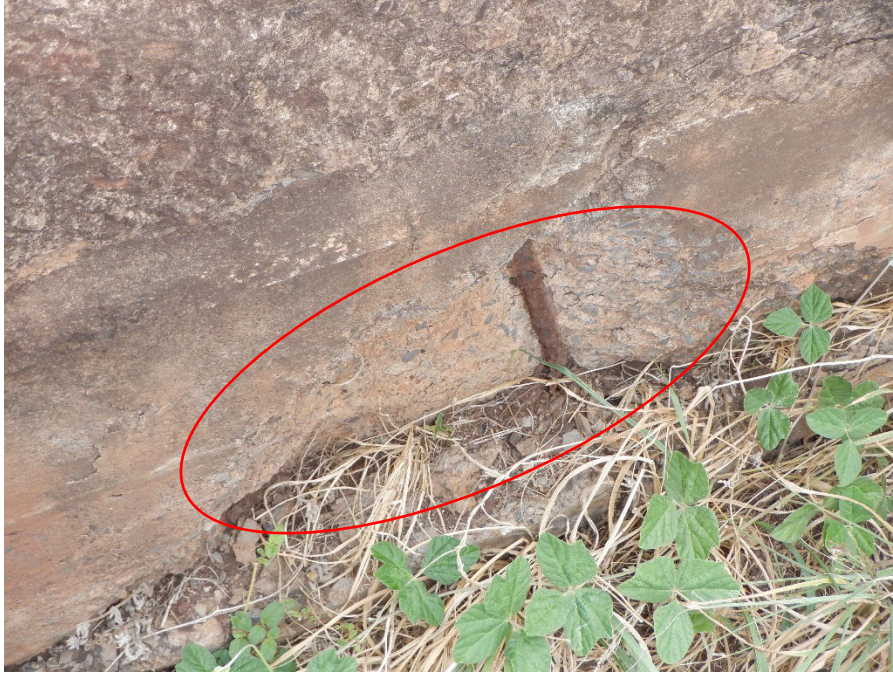
PHOTO 17 1'X1'X2" SPALL WITH EXPOSED REBAR WITH 0.31 SQ. IN SECTION LOSS (1FT 1090 CS3) ON INTERIOR FACE OF UPSTREAM RAILING, 12' FROM NORTH END OF BRIDGE
