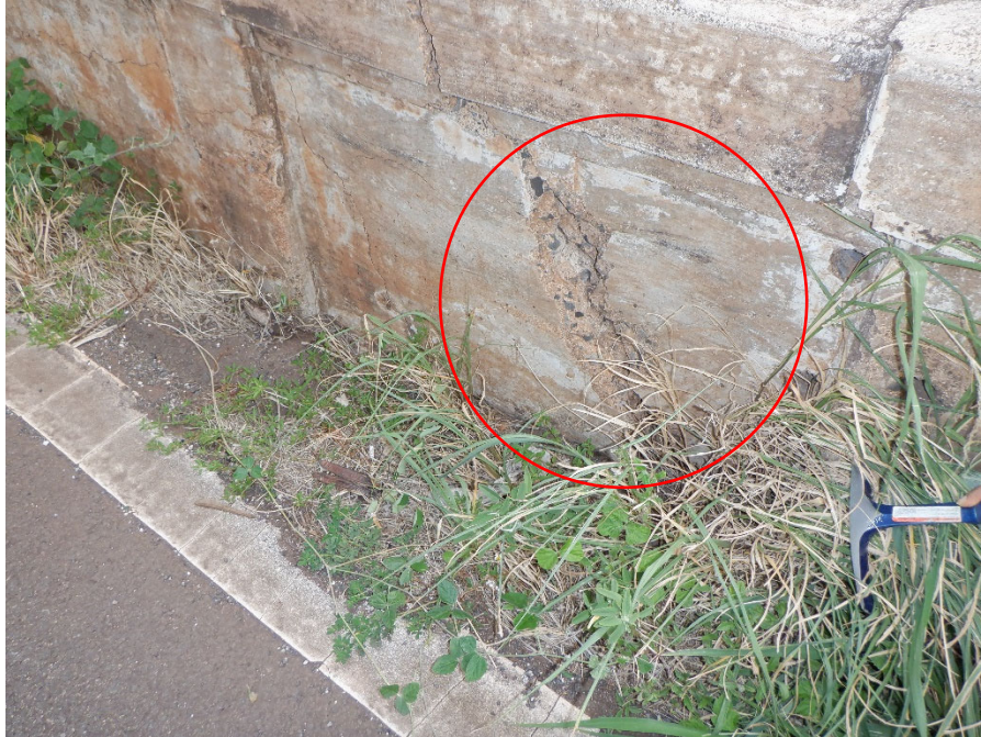
PHOTO 11 9"X1'-8"X2-1/2" SPALL (1FT 1080 CS3) ON INTERIOR FACE OF UPSTREAM RAILING, 2' FROM NORTH END OF BRIDGE
