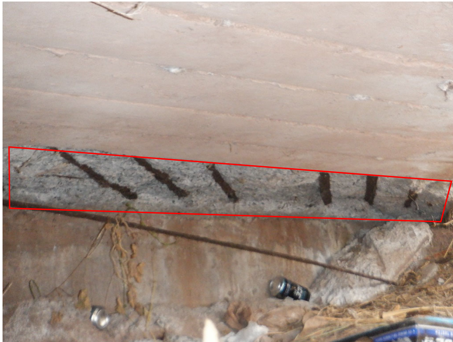
PHOTO 28 8'X3' SPALL WITH EXPOSED REBAR WITH 0.0123 SQ. IN SECTION LOSS (24SF 1090 CS3) ON SLAB SOFFIT ALONG ABUTMENT 2 STARTING FROM DOWNSTREAM END
