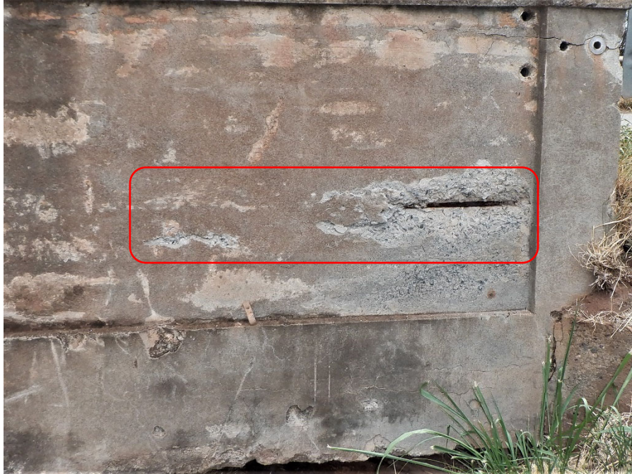
PHOTO 13 4'X1'-6"X2" SPALL WITH EXPOSED REBAR (4FT 1080 CS3) ON EXTERIOR FACE OF UPSTREAM RAILING, 2' FROM SOUTH END OF BRIDGE
