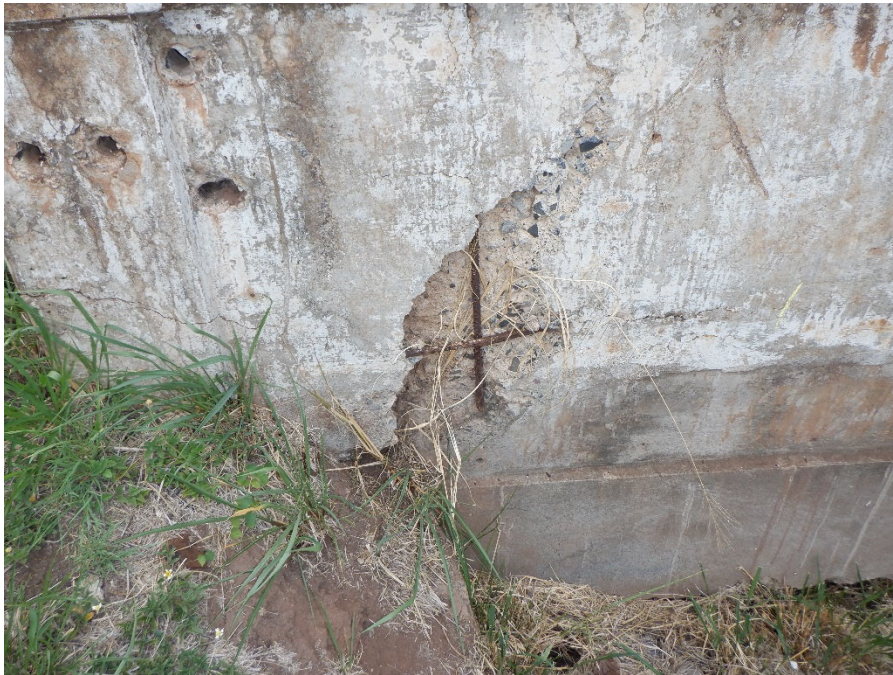
PHOTO 10 3'X3'X4" SPALL WITH EXPOSED REBAR (3FT 1080 CS3) ON EXTERIOR FACE OF UPSTREAM RAILING, 2' FROM NORTH END OF BRIDGE
