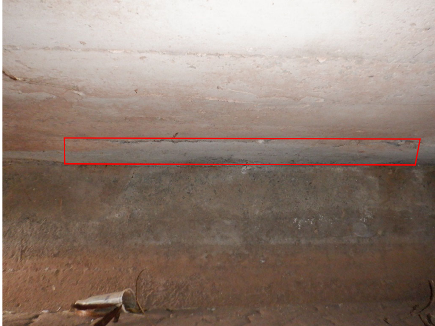
PHOTO 23 8'X2' DELAMINATION (16SF 1080 CS3) ON SLAB SOFFIT ALONG ABUTMENT 1, 5' FROM DOWNSTREAM END
