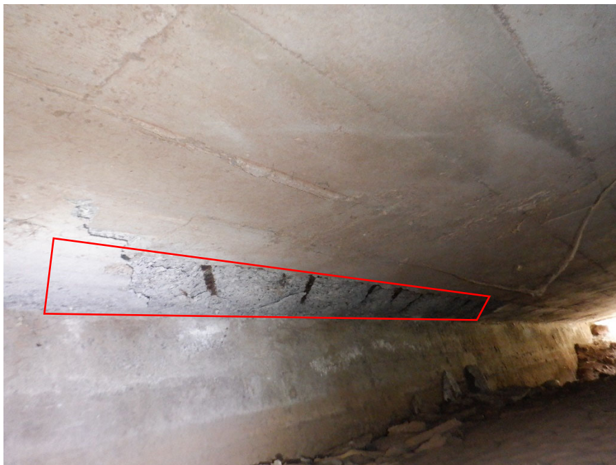
PHOTO 26 12'X2' SPALL WITH EXPOSED REBAR WITH 0.0123 SQ. IN SECTION LOSS (24SF 1090 CS3) ON SLAB SOFFIT ALONG ABUTMENT 1, 10' FROM DOWNSTREAM END
