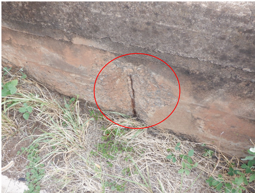
PHOTO 16 1'X1'-6"X2" SPALL WITH EXPOSED REBAR WITH 0.31 SQ. IN SECTION LOSS (1FT 1090 CS3) ON INTERIOR FACE OF UPSTREAM RAILING, 10' FROM NORTH END OF BRIDGE
