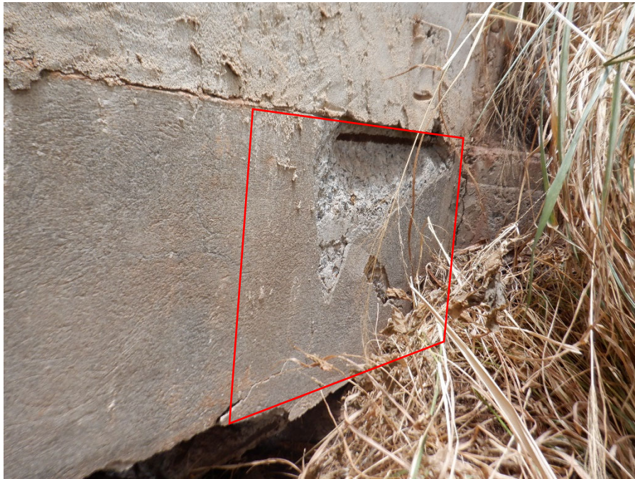
PHOTO 24 2'X2' DELAMINATION AND SPALL WITH EXPOSED REBAR (4SF 1080 CS3) ON DOWNSTREAM FACE OF SLAB AT ABUTMENT 2
