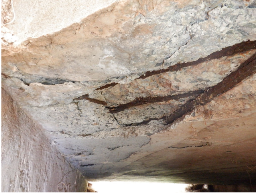
PHOTO 25 2'X2' SPALL WITH EXPOSED REBAR WITH 0.0123 SQ. IN SECTION LOSS (4SF 1090 CS3) ON SLAB SOFFIT AT DOWNSTREAM END OF SLAB SOFFIT ADJACENT TO ABUTMENT 1
