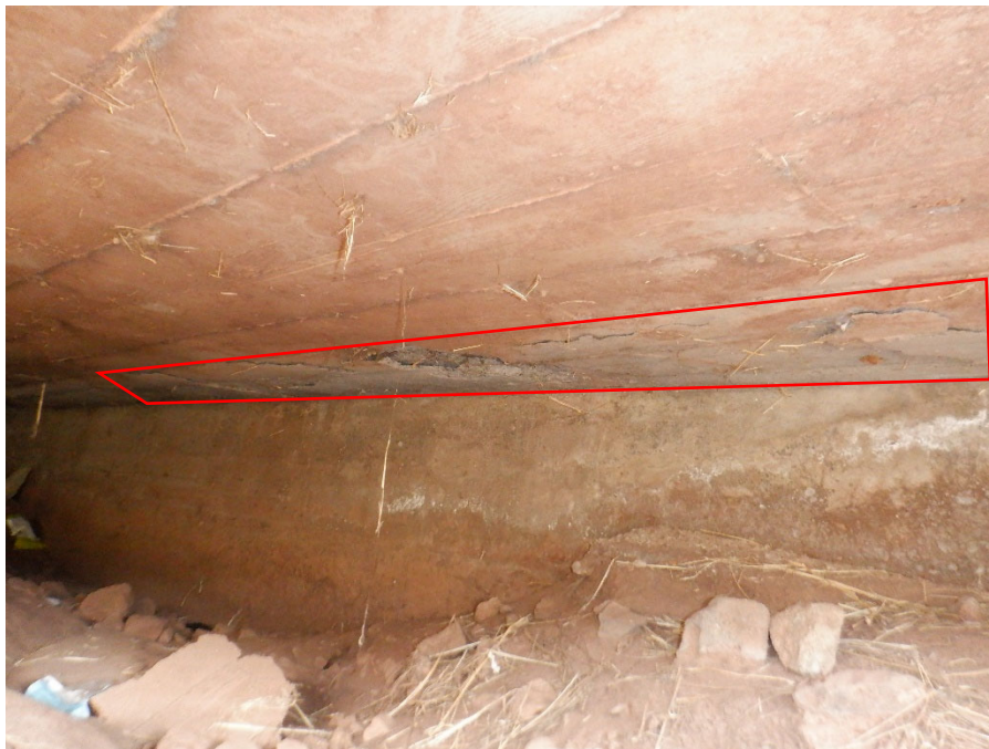
PHOTO 22 14'X2' DELAMINATION (28SF 1080 CS3) ON SLAB SOFFIT ALONG ABUTMENT 1 STARTING FROM UPSTREAM END
