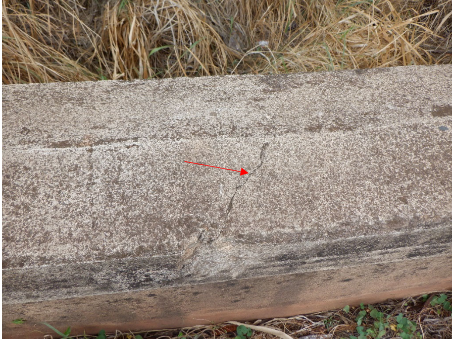
PHOTO 19 TYPICAL MODERATE WIDTH CRACK (1130 CS2) ON BOTH BRIDGE RAILINGS
