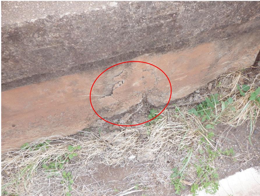
PHOTO 18 1'X1'-6"X2" SPALL WITH EXPOSED REBAR WITH 0.31 SQ. IN SECTION LOSS (1FT 1090 CS3) ON INTERIOR FACE OF UPSTREAM RAILING, 14' FROM NORTH END OF BRIDGE
