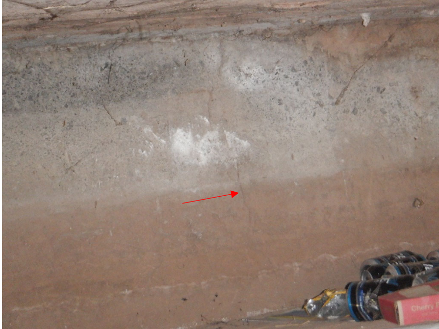
PHOTO 31 MODERATE WIDTH VERTICAL CRACK (1FT 1130 CS2) ON ABUTMENT 2
