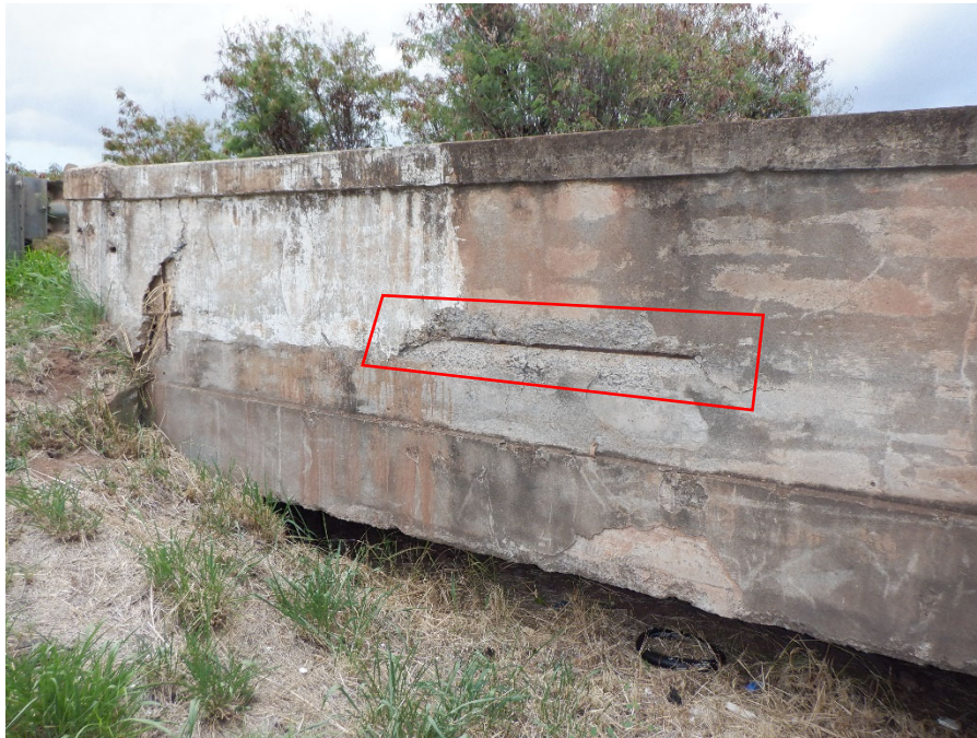
PHOTO 12 5'-3"X1'-6"X3" SPALL WITH EXPOSED REBAR (6FT 1080 CS3) ON EXTERIOR FACE OF UPSTREAM RAILING, 10' FROM NORTH END OF BRIDGE
