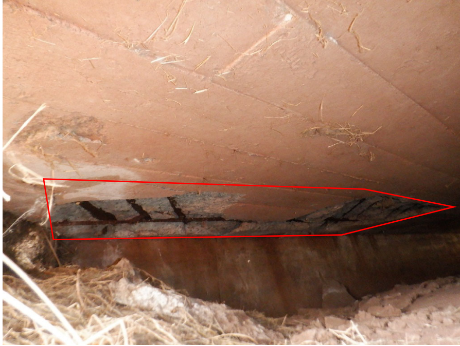
PHOTO 27 10'X2' SPALL WITH EXPOSED REBAR WITH 0.0123 SQ. IN SECTION LOSS (20SF 1090 CS3) ON SLAB SOFFIT ALONG ABUTMENT 2 STARTING FROM UPSTREAM END
