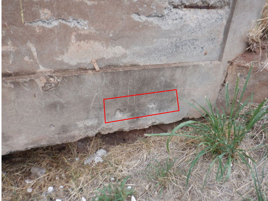
PHOTO 21 3'X1' DELAMINATION (3SF 1080 CS3) ON UPSTREAM FACE OF SLAB ADJACENT TO ABUTMENT 1
