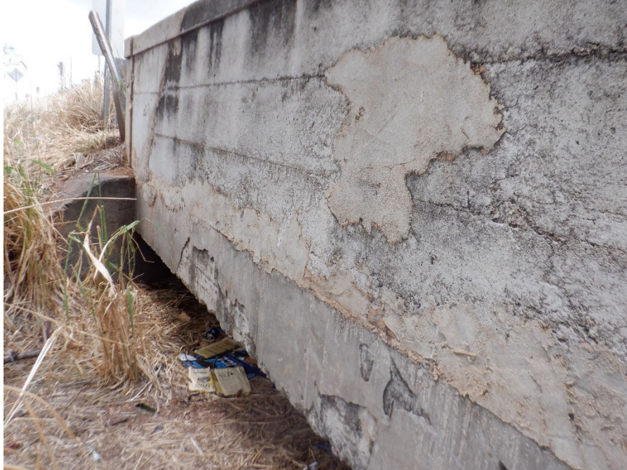
PHOTO 15 TYPICAL SOUND CONCRETE PATCHES (8FT 1080 CS2) ON EXTERIOR FACE OF DOWNSTREAM RAILING
